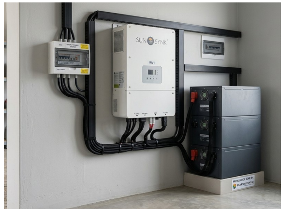
Inverter and battery storage systems
